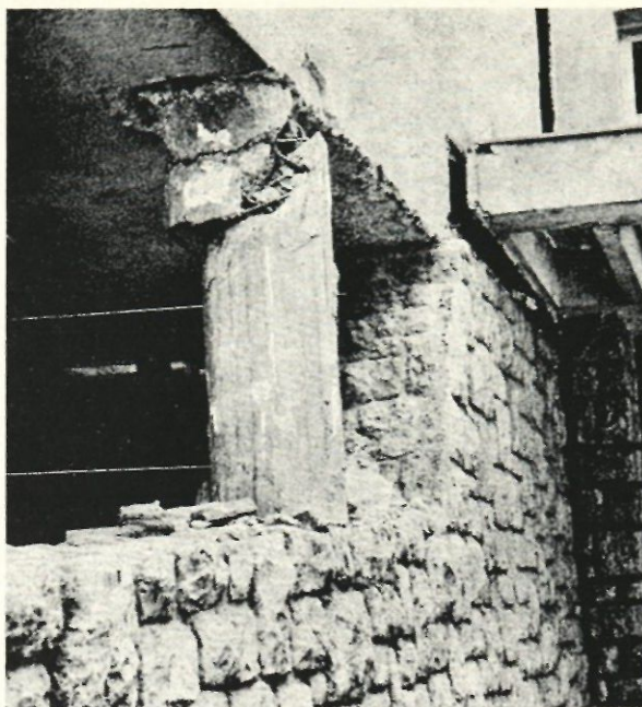
Figure 5: Column Shear Failure (2.58) (Courtesy of American Iron and Steel Institute.)
