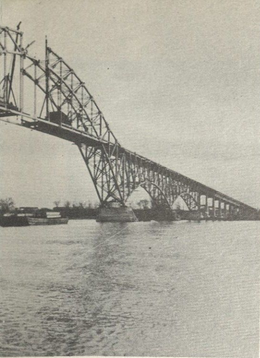
—Courtesy American Inst. of Steel Construction of the South Grand Island Bridge. A traveling, stiff- the top of the towering channel span.
