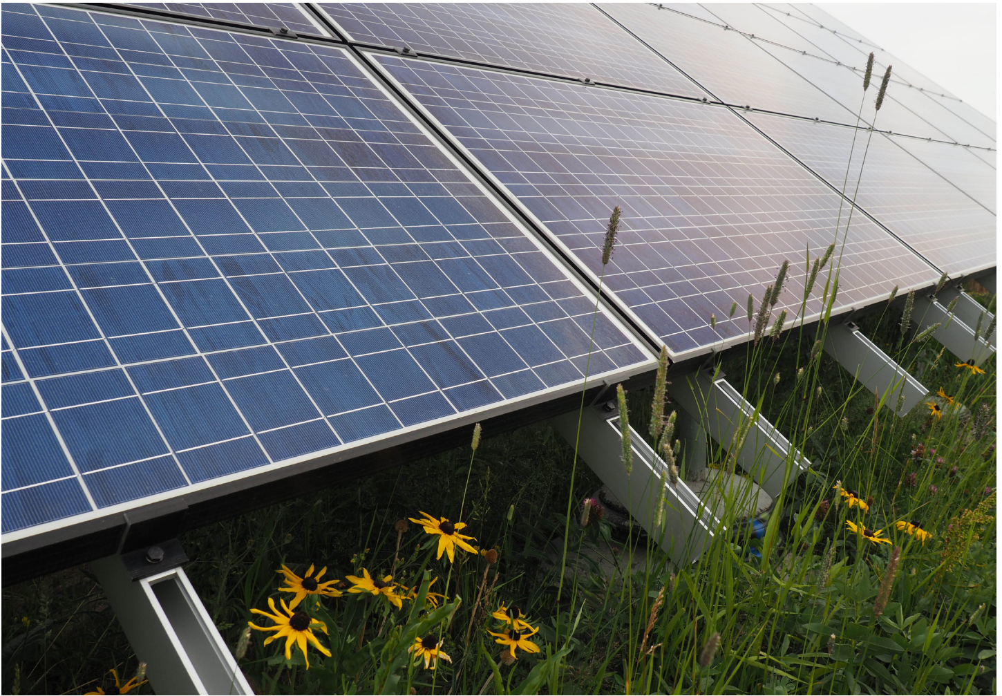
Wildflowers bloom near solar panels on Niwot Ridge in Boulder County, Colorado. (Jeff Lukas/CIRES)
