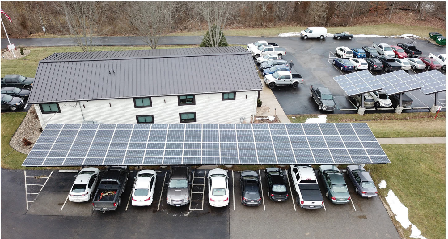
Pickering Associates' carport structure and 4 EV charging stations; 40kW solar, Parkersburg, West Virginia. (Kelly Bragg / West Virginia Clean Cities / NREL 61267)
