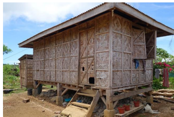
Shelter materials show signs of wear.
