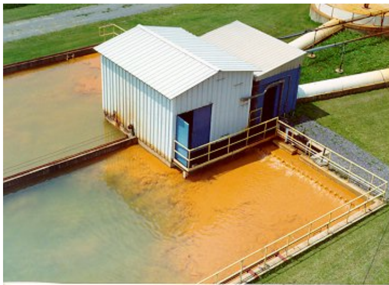
A settling pond for the treatment of acid mine drainage.
