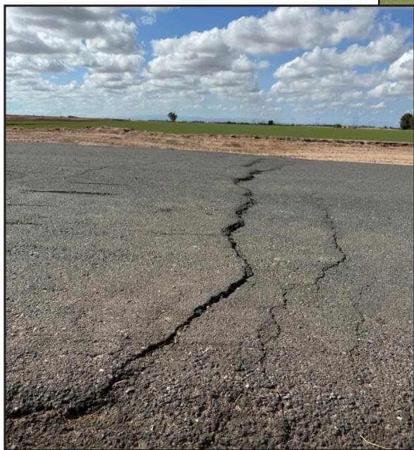
A view of the Brawley Fault Zone where it crosses Harris Road in Imperial County, CA, and produces a sharp break in the pavement. The Brawley fault is an oblique right-lateral/normal fault in the Imperial Valley with a slip rate of several mm/yr. This view is to the south, and the hanging wall of the normal fault is on the right (west) side. This fault ruptured in a M6.5 earthquake in 1979 and has been creeping episodically in the years since. photo credit: Kathryn Materna
