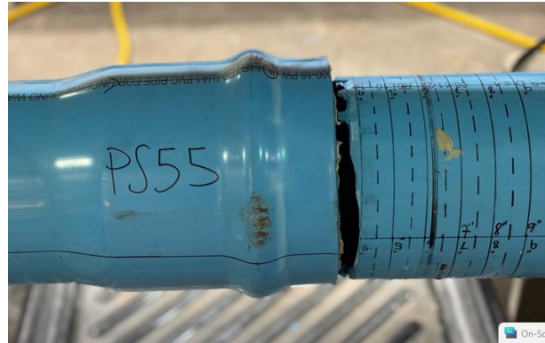
Figure 4.44. PS55 joint failure due to fracture on the spigot
