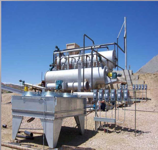
EnShale Pilot Plant in Utah
