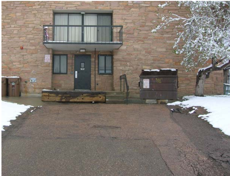
Deteriorated paving and cosmetic issues
