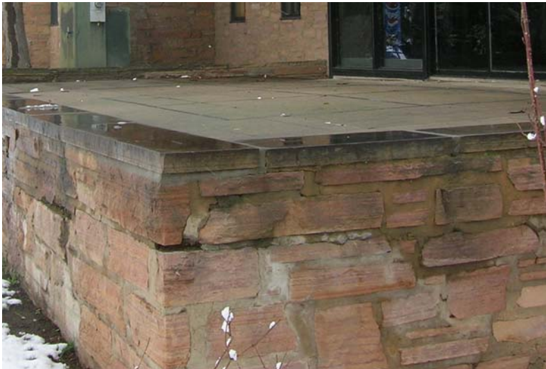
Site wall with deteriorated mortar joints
