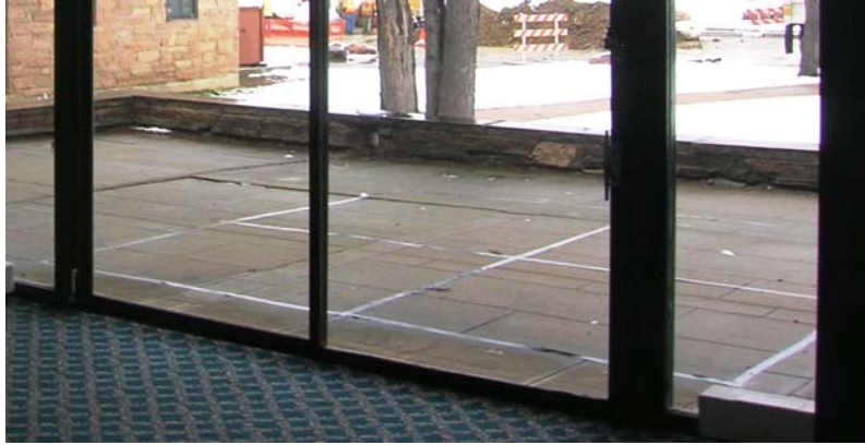
Terrace paving problems
