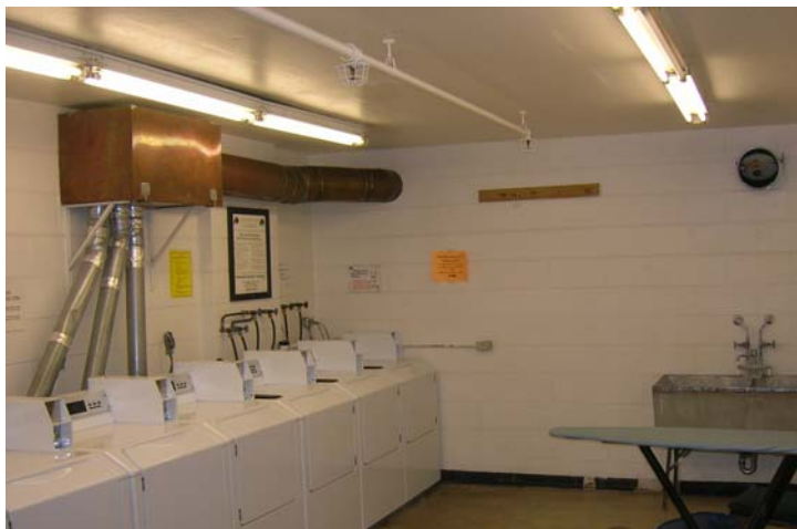
Exposed Building Systems
