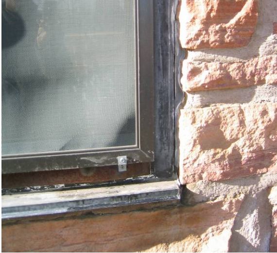
Windows show deterioration
