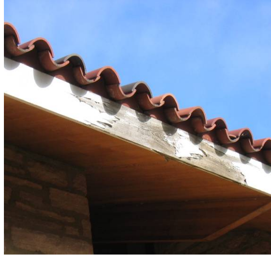
Fascia repair/repaint required at Andrews
